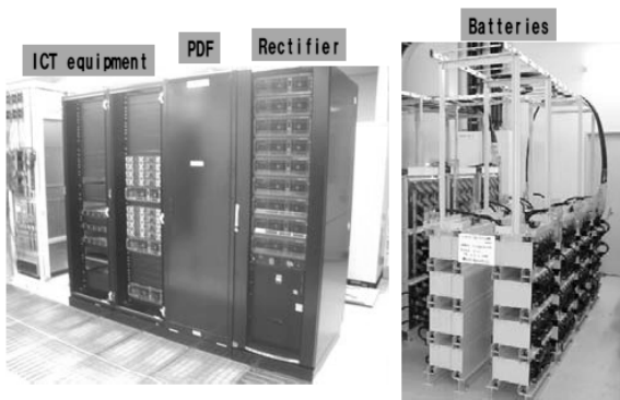
Fig. 28 Overview of the 380 VDC power supply system.
